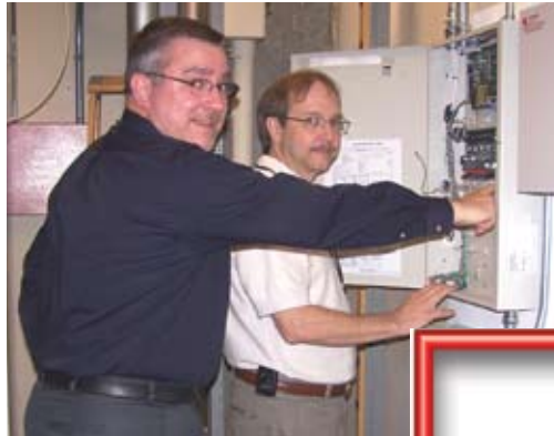
Left: Guerry Bruner (left) of Tech Systems and Tom Morris (right) of Georgia Power inspect one of the many Software House iSTAR Network Controllers located throughout Georgia Power.
