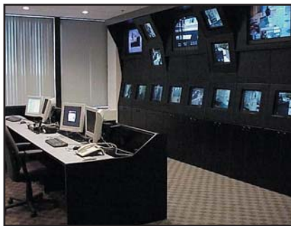
The control center from one of Peter Barry's large projects.
